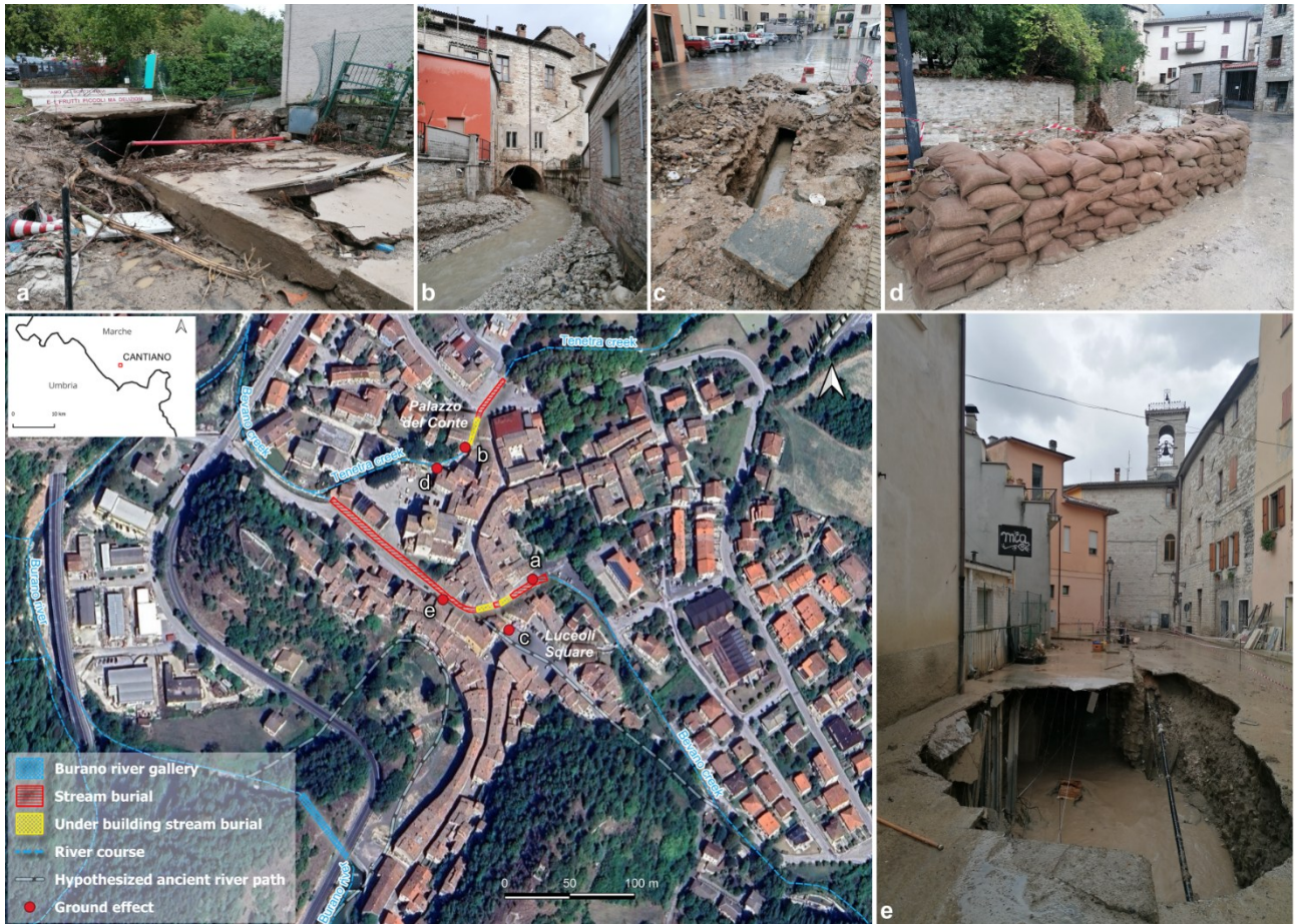
Fig. 4. Location of the effects of the high flow rates in the artificial stretch of riverbeds and sewer system within the built-up area of Cantiano. (a) pavement and road torn off by the overflowing water of the Bevano creek; (b) outlet of the underground river bed of the Tenetra stream and related material transported; (c) break in the sewerage network in front of the Municipality; (d) natural protections set up during the emergency; (e) breaking point of the culvert caused by the high hydraulic pressure created.
