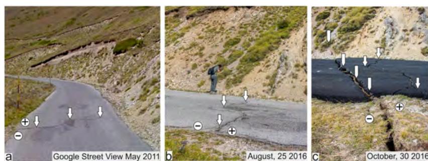
Figure 7. Multitemporal view of the coseismic ruptures in the asphalt pavement of the Strada Provinciale n. 477 on the southern slope of Mt. Vettore (see location in Figure 5); white arrows indicate the same location at different times; (a) Google Street View from May 2011 [81], where a small down-slope step is observable; (b) oblique image of the coseismic ruptures after 24 August 2016 event, during which the previous discontinuity was reactivated in the upslope; (c) oblique photo of the coseismic ruptures after the 30 October 2016 event, during which the reactivation of the previous fractures occurred and new fractures were generated (white arrows).
