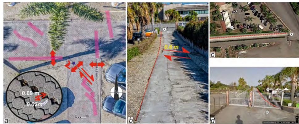
Figure 15. Ground ruptures formed during the 26 December 2018 seismic event along the Fiandaca fault (red arrows indicate the movement direction—cyan strips are the deformed zone—dashed red line indicate the undeformed lane edge): (a) displacement of interlocking bricks in a parking pavement (point y in Figure 14) associated with right lateral strike-slip motion; (b) displacement of a private lane surveyed in March 2019 (from point x to point k in Figure 14); (c) the same area without visible ground deformations in a Google Earth image of 21 July 2018 [92]; and (d) Google Earth Street View from point k (July 2018) [93].
