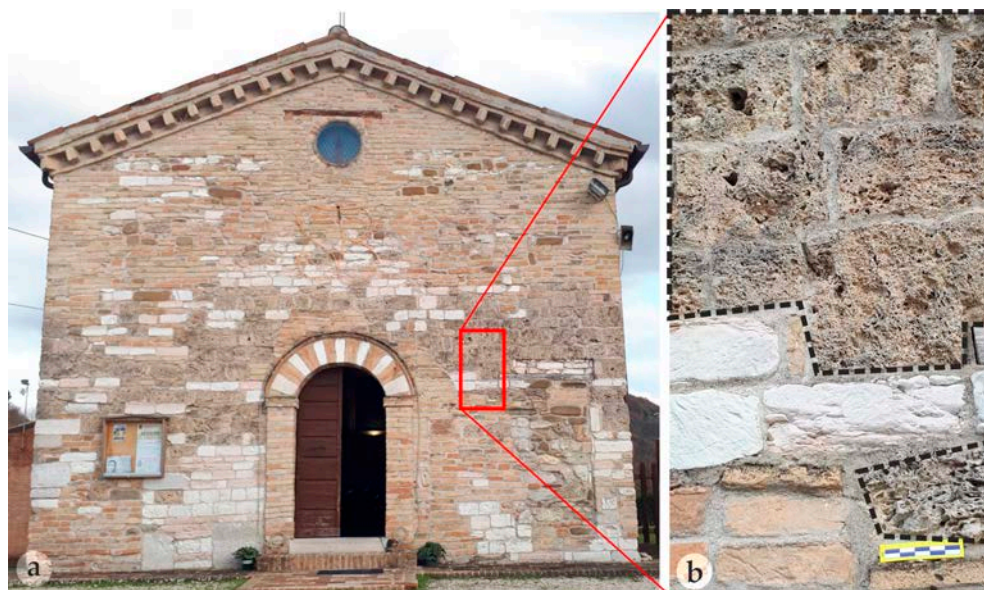
Figure 8. (a) Santa Barbara church (from the end of 12th to 14th century) partially built using calcareous tufas highlighted in the inset (b).
