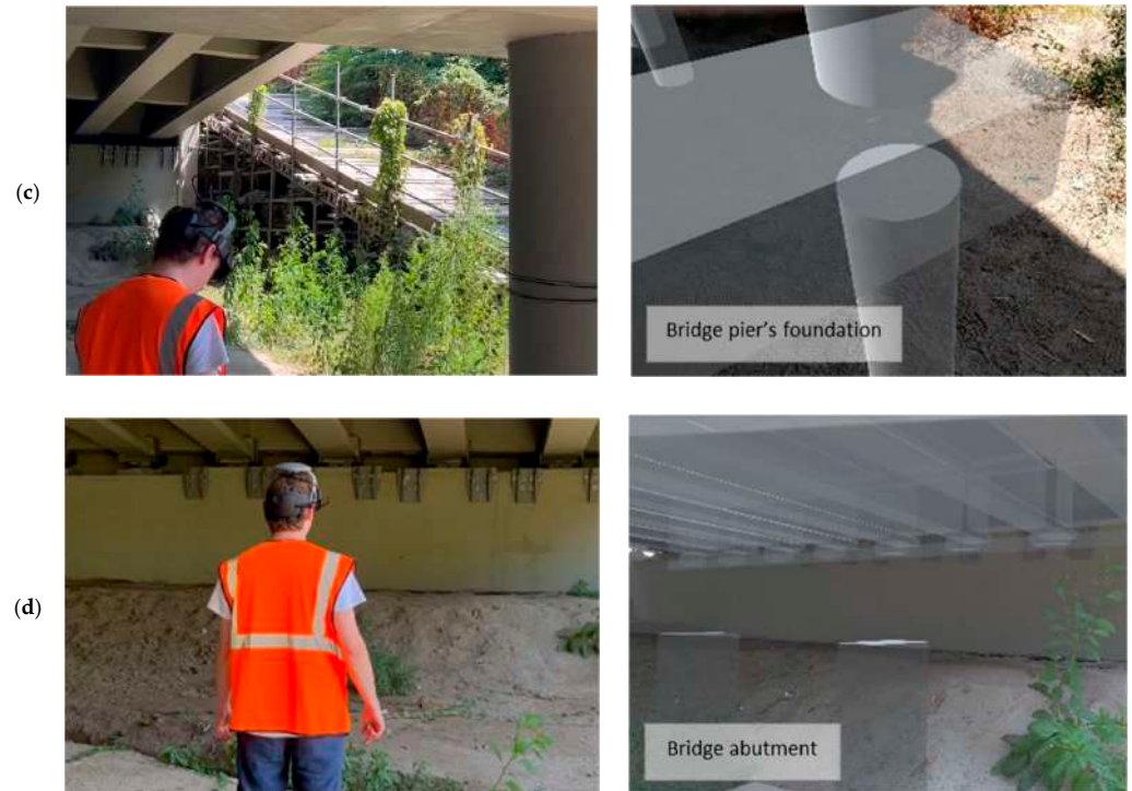
Figure 16. Stages of visual inspection of structural elements of the viaduct, including hidden bridge pier foundations: (a) visualization of the bridge from the open area; (b) visualization of the node between the bridge pier and the deck; (c) visualization of the foundation of the bridge pier; (d) visualization of the bridge abutment, its foundation, and the connection between the abutment and the deck.
