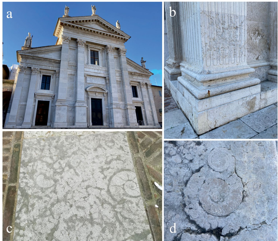
Fig. 9 Stop 6: the façade of the Cathedral mostly made of lithotypes of the Bugarone Group (a) characterised by degradation phenomena of detachment and staining due to pyrite oxidation (b); particulars of the square adjacent to the Cathedral, paved with bricks and blocks of the Bugarone Group characterised by big fossils of Ammonites (c, d)
